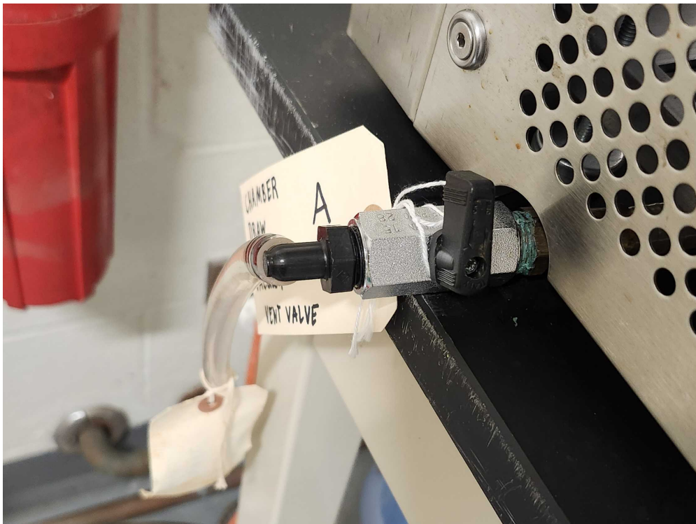
Drainage hose in the closed position
