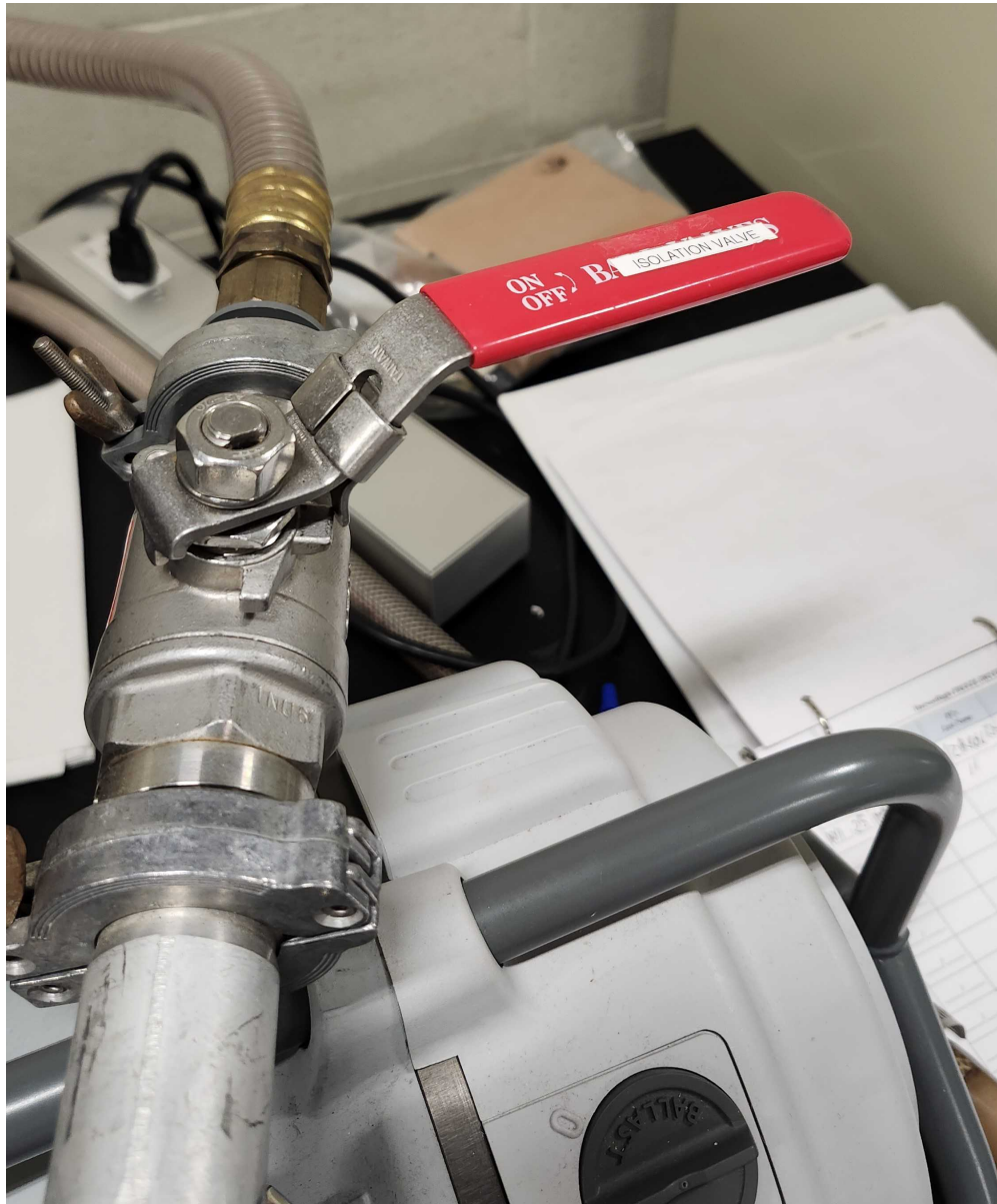
Vacuum pump in the partially open
