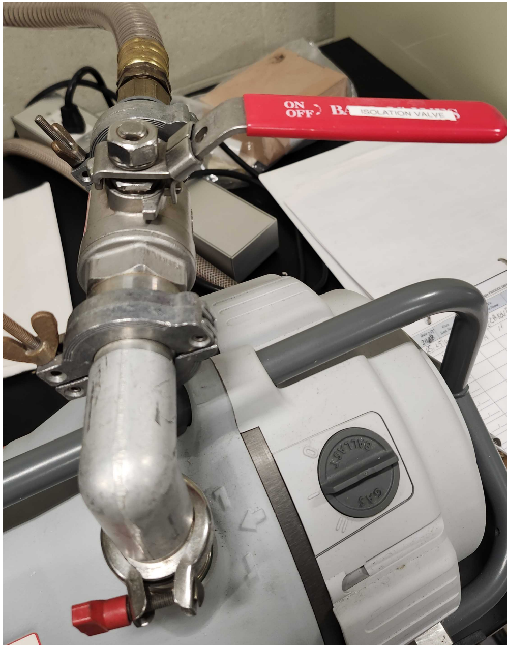
Vacuum pump in the closed position
